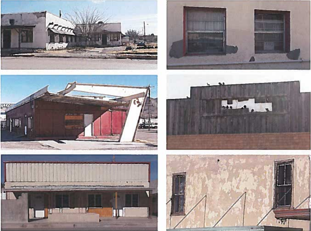
Photos showing a sample of building conditions in the MainStreet District
