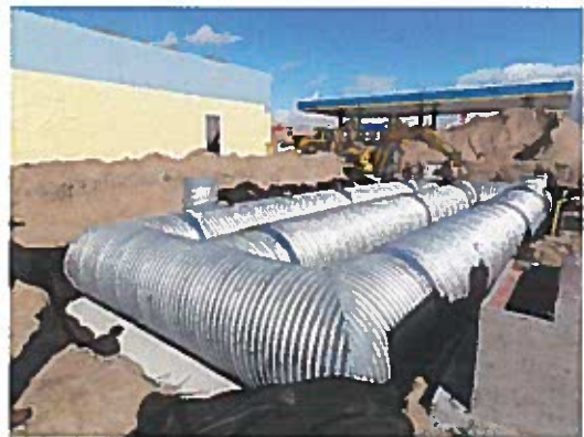
Underground storage of storm water.
